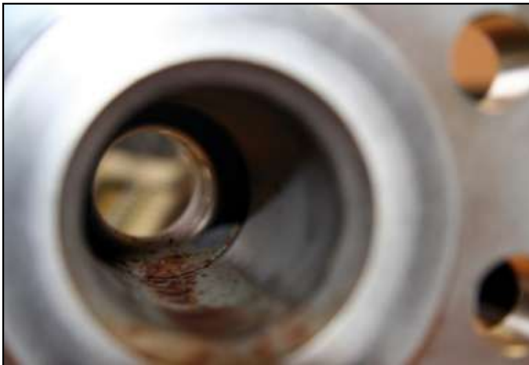
Figure 6: Internal condition of the eTube with a slight rust strip due to saline liquid stagnation
