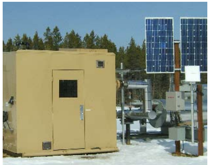
Satellite installation with control and many additional surface facility peripherals
